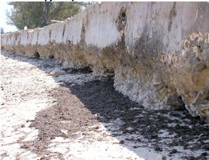
Severe scouring is associated with many Bahamian sea walls
