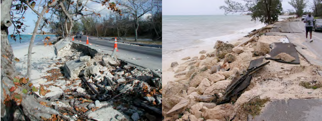
Sea wall failure at Caves Point, NP, after H Michelle (2001) and H Frances (2005)
