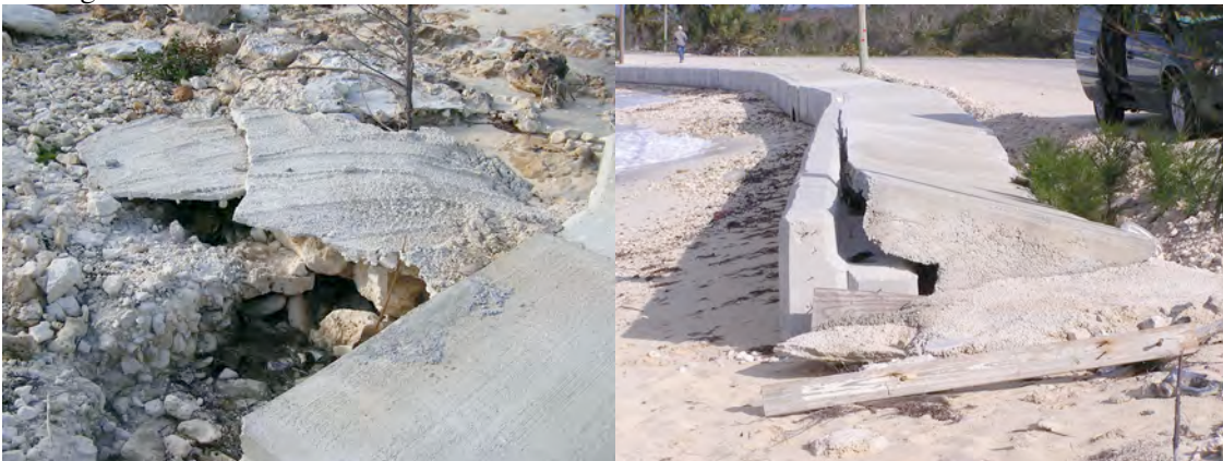
Improperly finished wall end; and wall collapse due wall end failure, both Cat Island.
