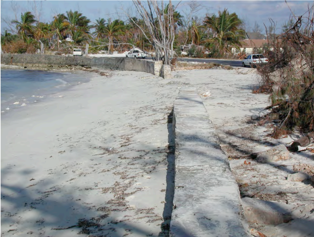
Breached sea wall at West Bay Street, New Providence.
